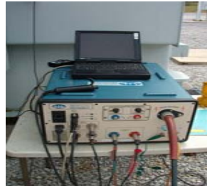
Power Factor Testing utilizing the Doble M-4000 Test Set
